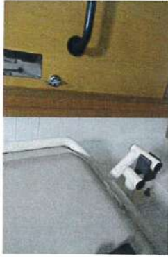
The space to the latch side of the door is obstructed by the baby change table.
